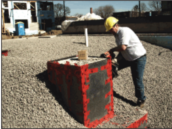
Building piers isolated from ground borne vibration. 1 - 3 layers of Iso-sep 25F for the base.
