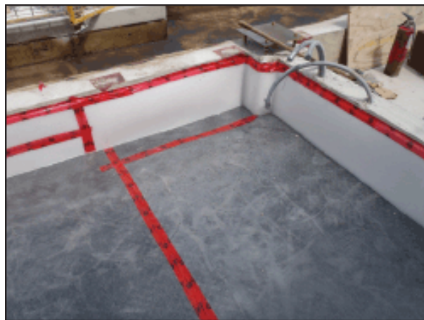
Non critical applications use single layer Iso-Sep 25HD and Perimeter Isolation Board. - Example: Pump Rooms
