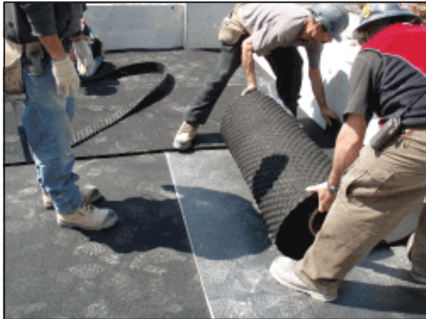
Critical applications use 2 layers Iso-Sep 25HD and Perimeter Isolation Board - example: Standby Generators over condo suites.
