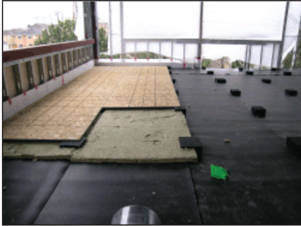
Building conversion floors using mass loaded vinyl to seal existing structure and a discrete isolator floating floor system.
